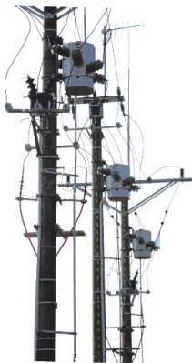
THO-24 load switches on poles.
